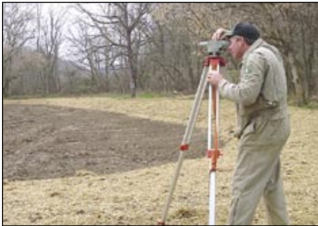
Using a level to measure slope on a vernal pond construction site.
