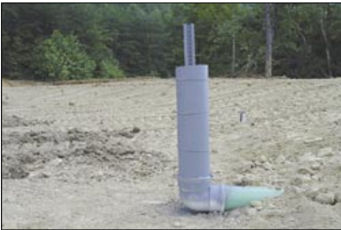
This PVC pipe serves as an overflow pipe when vertical; the stake provides support to the pipe.
