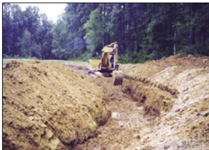
As the trench is being dug, silt loam is placed inside the wetland; gravel outside the wetland.
